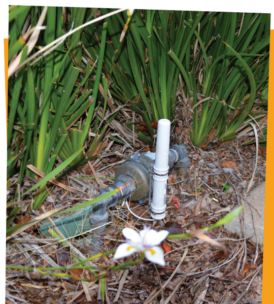
Water meter retro-fitted with a remote meter reading unit
