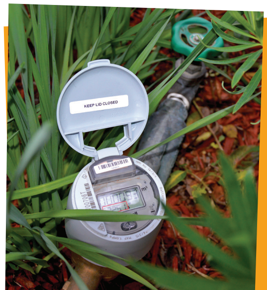
Old water meter replaced with a remote meter
